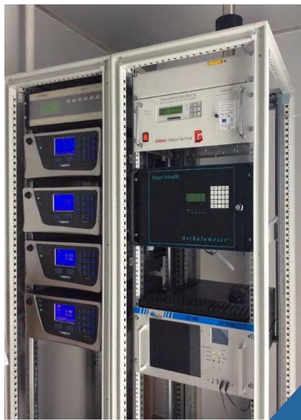
Air Quality monitoring equipment
