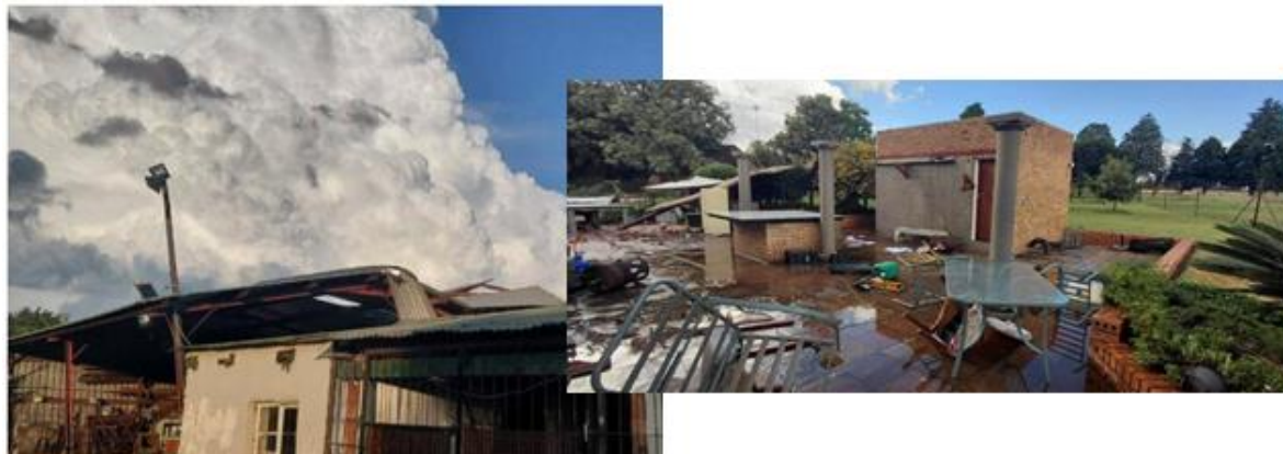
Figure 1: A recent supercell thunderstorm that caused a brief tornado with strong damaging winds to the north-east of Middelburg (Pictures: © Middelburg Observer)
