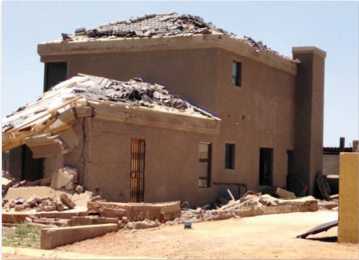
Figure 7: One of the houses in Protea Glen, Soweto, that was severely damaged by the tornado that occurred on 30 December 2017. Photo: © P. Mofokeng, 2017.
