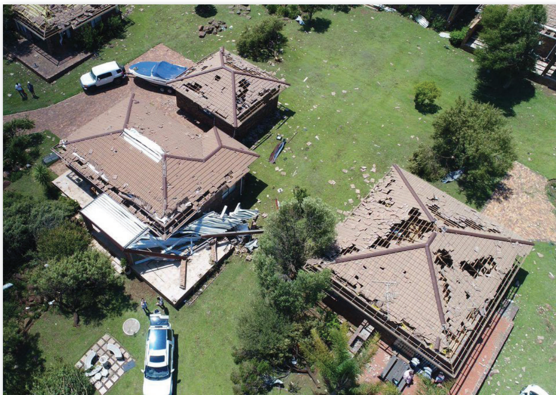
Figure 9: Aerial photo of storm damage to property at Vaal Marina following the 11 December 2017 tornado. Photo: © Brett Powell, 2017.
